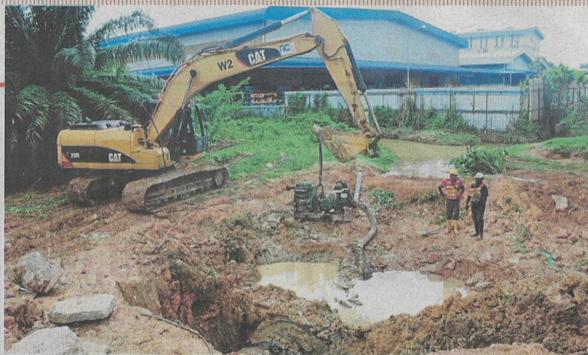
Repair works being carried out on a burst pipe in Setia Alam, Shah Alam, yesterday. BERNAMA PIC
